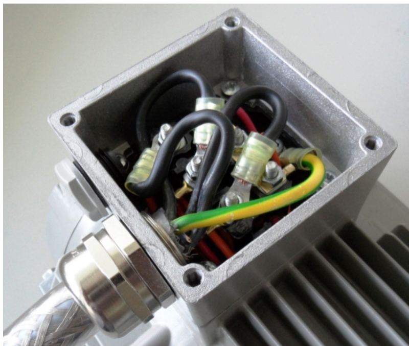
Fig. 26: Wiring on the motor connection box
